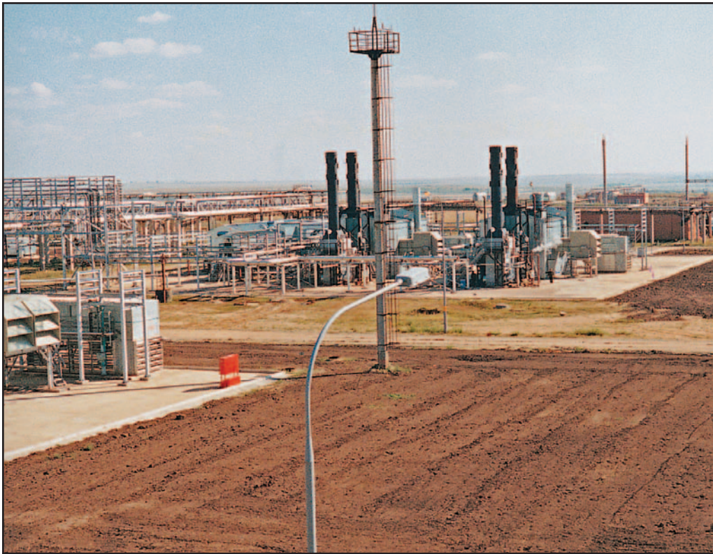
■ A 10 MW power generation and distribution plant was fabricated by TDE for OrenburgNeft in southwest Russia.
