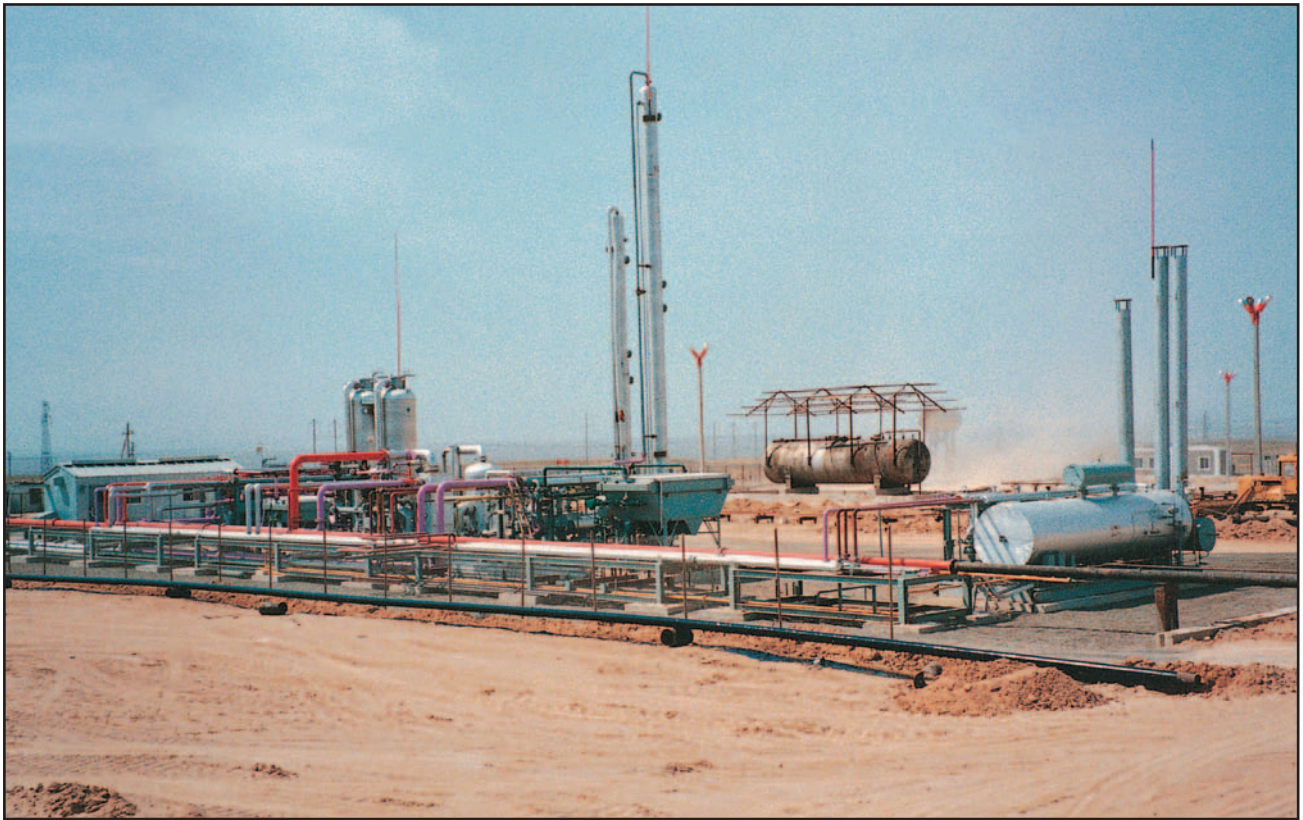
■ TDE is currently fabricating the third train of a grassroots LPG recovery plant for Turkmenistan. The new train will be similar to Trains 1 and 2 that are already installed and operational.
